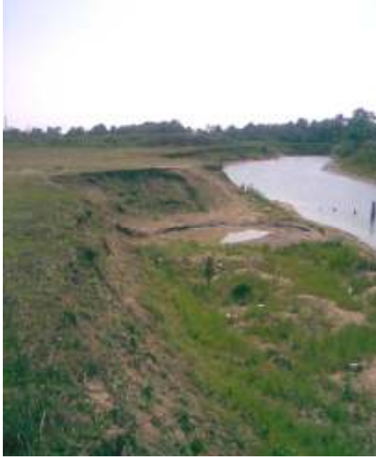
Figure. 1.6 Advanced erosion on the right bank of the meander
